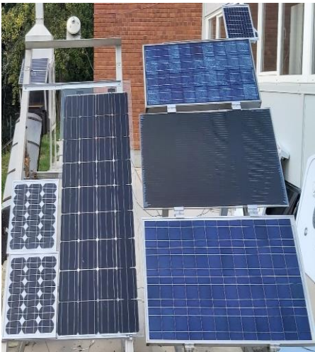
Fig. 2. Installed PV modules
