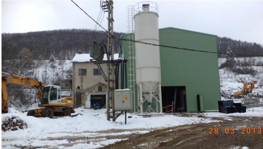
Figure 3. Establishing the water treatment station, till the old laboratory is standing this time (Recsk, Mining Site I-Lahóca, 28/03/2013)
